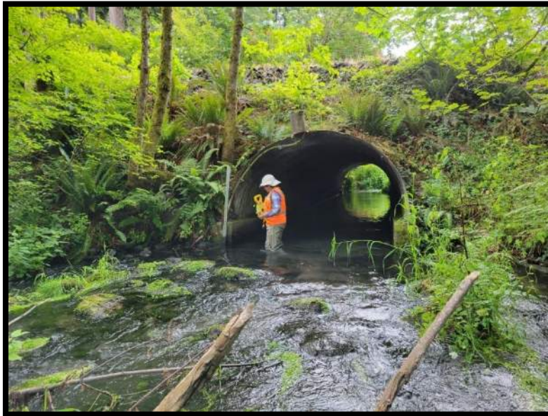
Figure 11: Culvert outlet at Draham St NE, facing upstream, approximately 25 feet downstream of the culvert outlet
