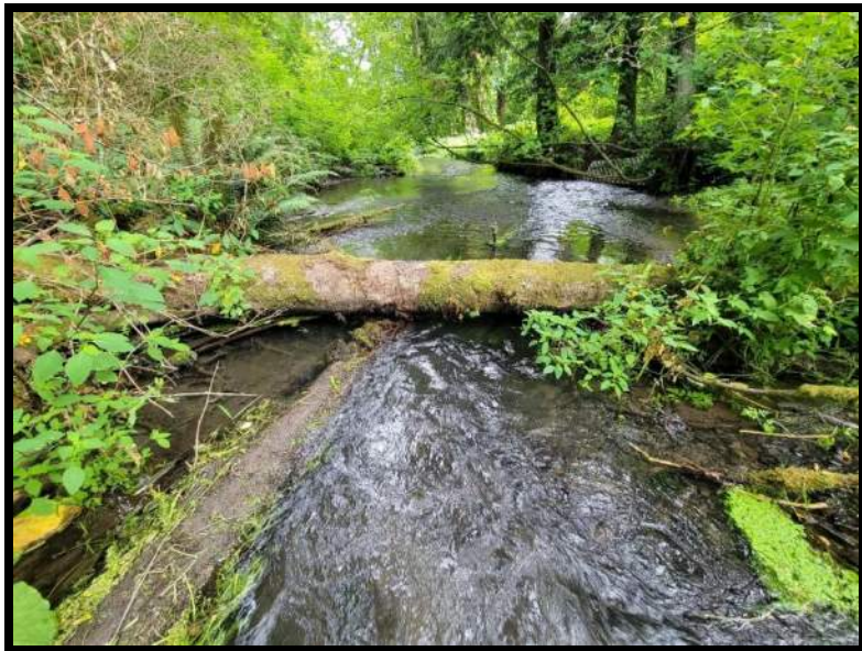
Figure 13: Large woody material accumulation approximately 160 feet downstream of the culvert outlet
