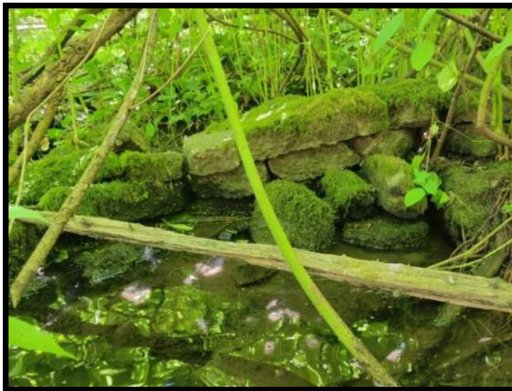
Figure 9: Concrete debris from abandoned weir forming obstruction in the channel approximately 50 feet upstream of the culvert inlet
