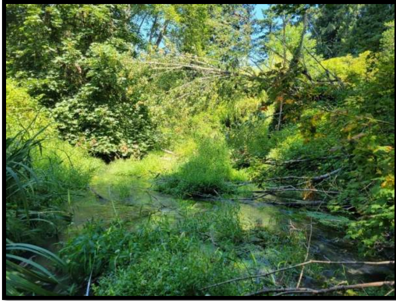
Figure 6: Woody debris and grass in the channel approximately 200 feet upstream of the culvert inlet
