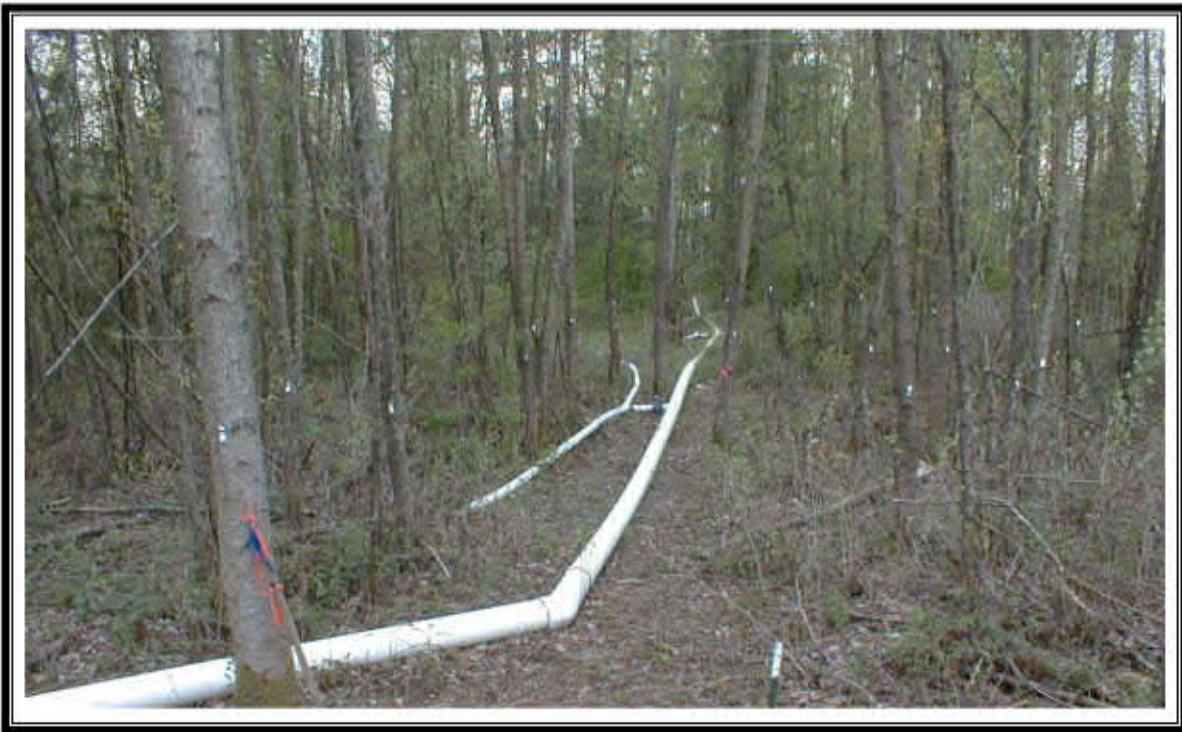
Figure 5.23. Manifold and Branches in a Wooded, Vegetated Spray Field.
