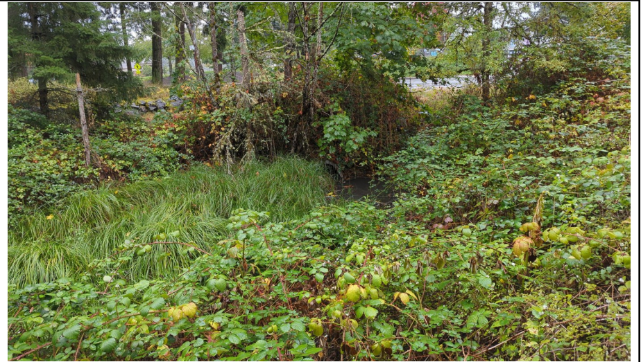
Photo 10. Facing south from the west side of the vegetated storm pond. The outlet culvert is shown in the center of the photo, on the south end of the pond. It is not known where the culvert leads to. October 2024.
