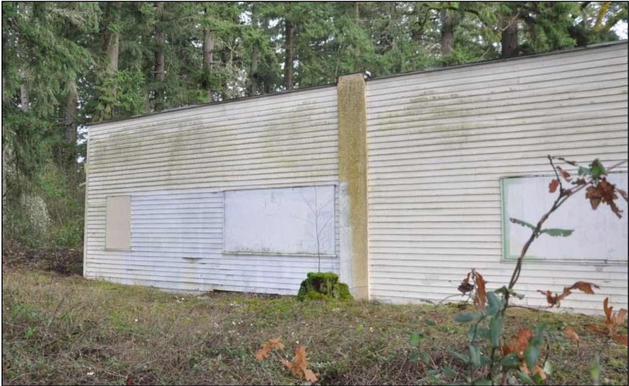
Photo 19. West façade with boarded up windows, view from southwest, taken in 2025.
