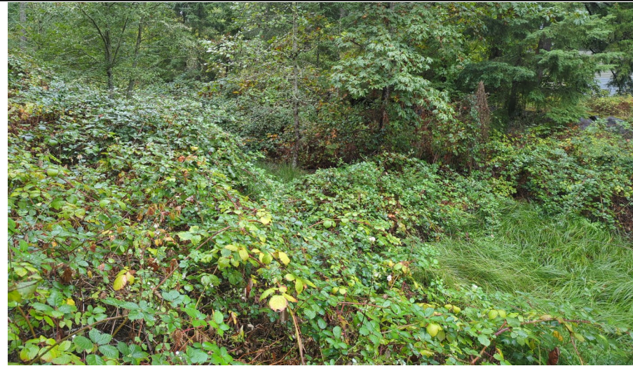
Photo 9. Facing north from the west side of the vegetated storm pond. The storm-pond is vegetated with a Carex species and Himalayan blackberry. October 2024.
