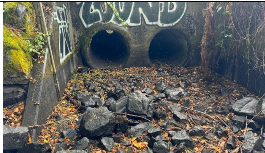
Photo 6. Facing southeast from the channel of Woodland Creek in the southern-most portion of the study area. The culverts are four feet in diameter and they span Pacific Avenue SE. October 2024.
