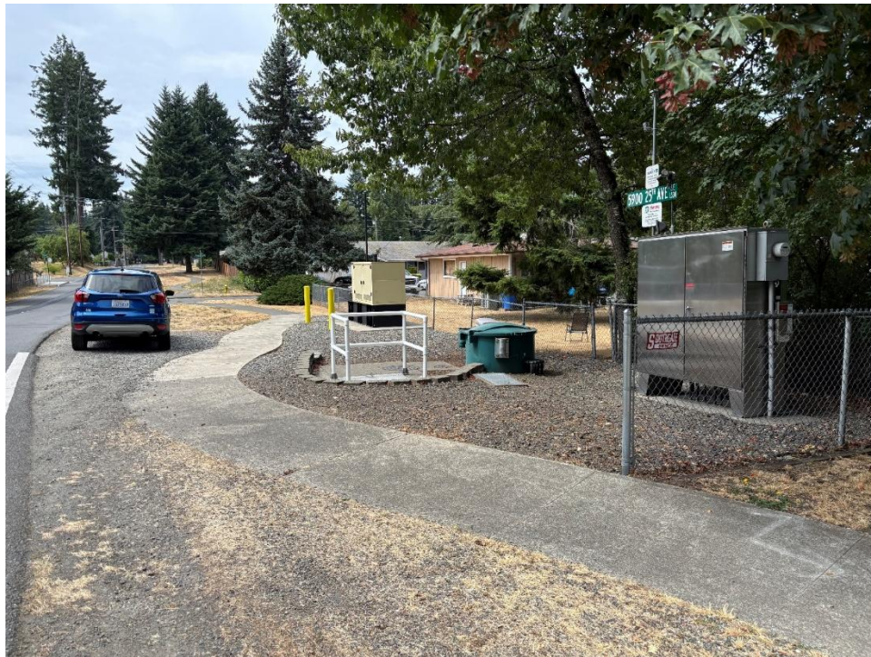
Existing LS4 looking West
