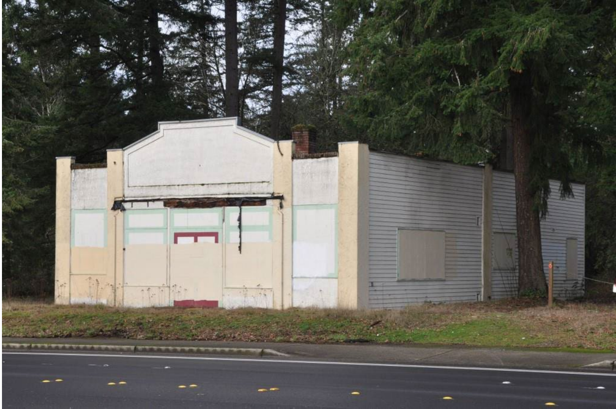
Photo 17. Current condition (2025) of the McKinney House, boarded over windows and doors.
