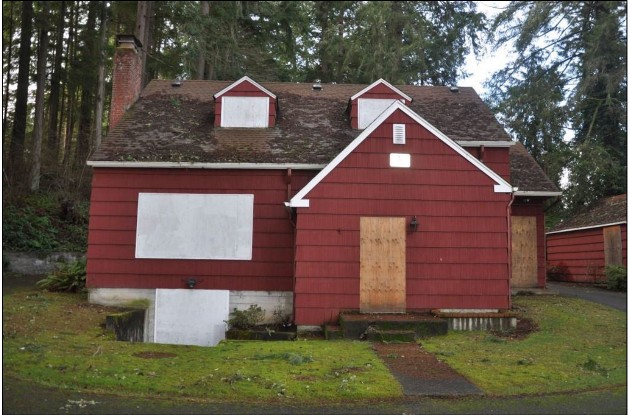
Photo 12. View of main (east) façade, note infill of windows and doors. Taken in 2025.
