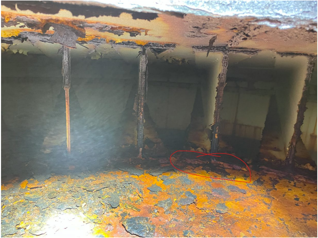
Figure 4: Central Column Corrosion
