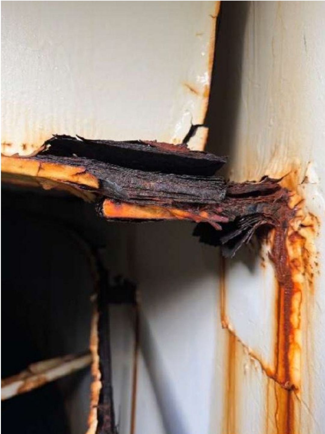
Figure 3: Rafter – Shell Connection Corrosion
