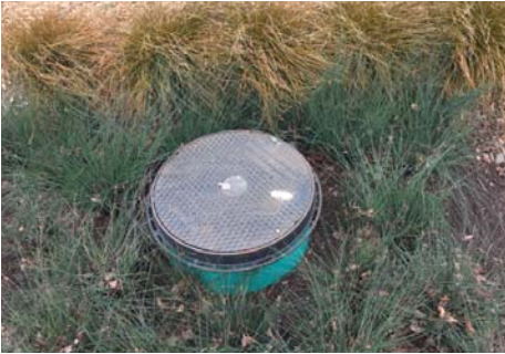
Underground Injection Control (UIC) Well
