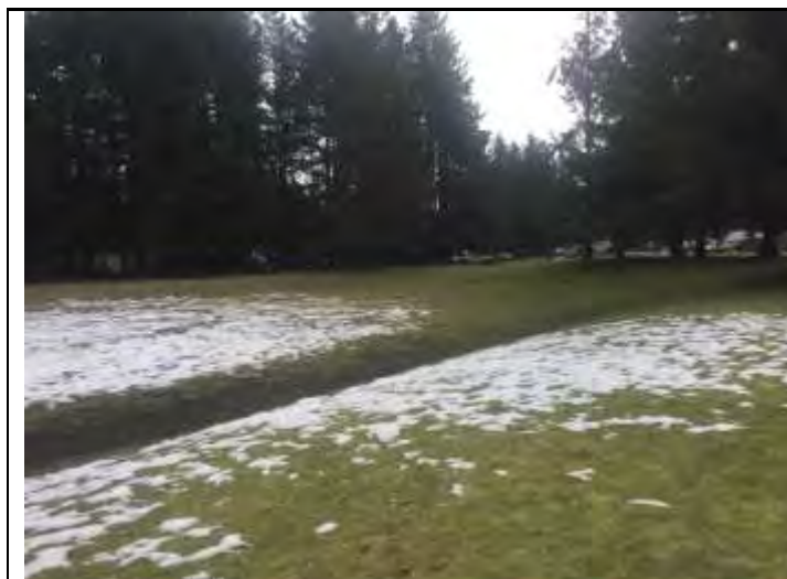
Evidence of ponding in low spots
